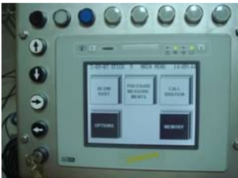
Panel for dust blowing
